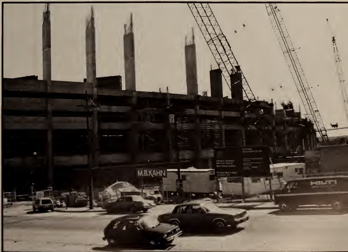
New deck construction started on Nov. 17, 1982 and ended at 10:46 pm, Friday, September 2, 1983.
